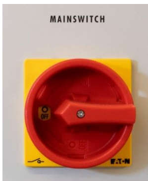
Figure 6: main switch 400V
